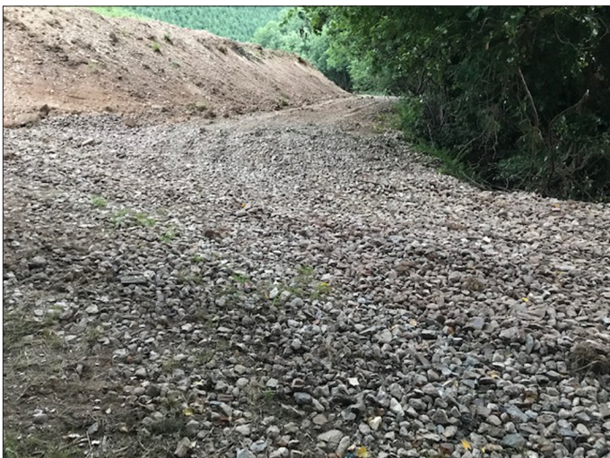
Soil heaped next to where the track has been cut in to the field
